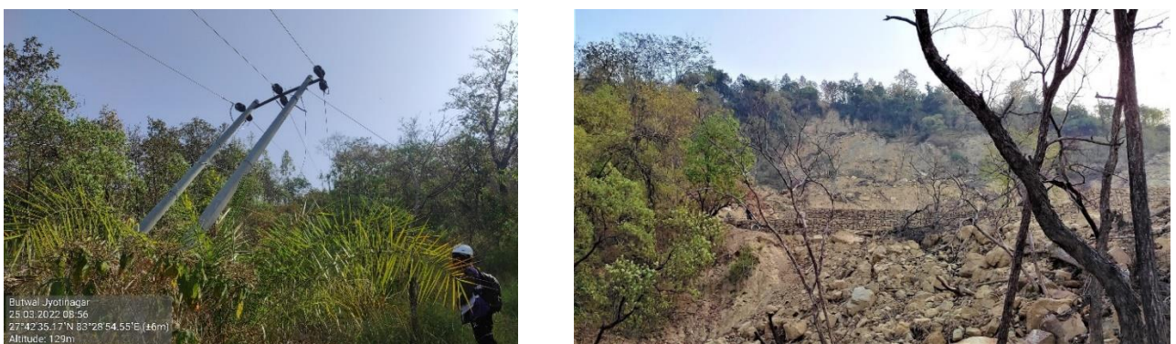
Figure 4 Tilted poles and gabion wall in the landslide area
