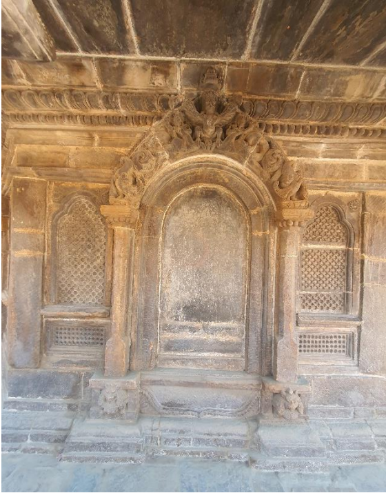
Figure 4: Entire wall including windows and door as well as the roof made with carved sandstone in the Chyasin Dewal temple of Patan Durbar Square
